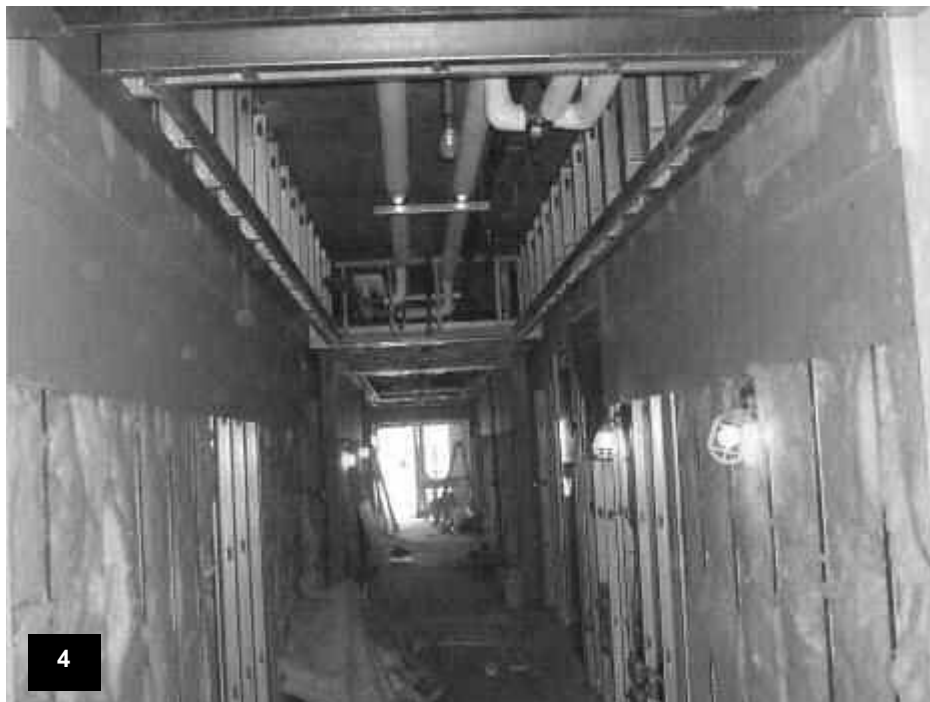
Tower Level T39 – View of the following in the main corridor; installed insulation, gypsum board along the ceiling, metal stud framing of the ceiling, main sprinkler line with sprinkler head stub-outs and electrical rough-in.
