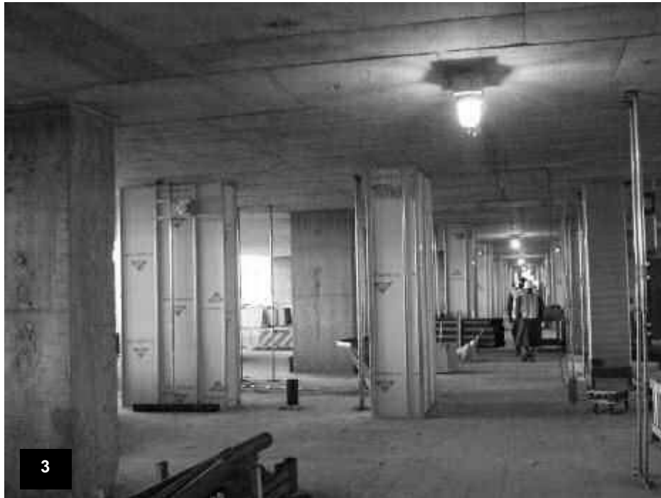
Tower Level T62 – View of the following: domestic hot and cold water supply lines, floor stub-up for the main sanitary sewer line, metal stud framing around the mechanical chases and mechanical chase branch line stub-out.
