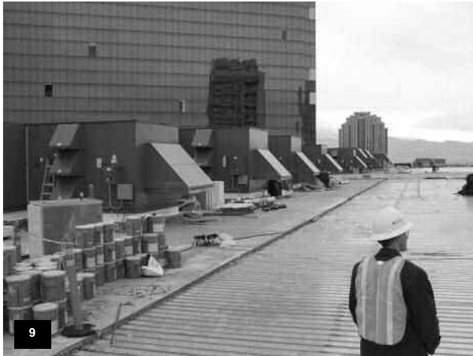
Garage/Convention Center – View of the roof top equipment located on the upper roof of the garage/convention center.
