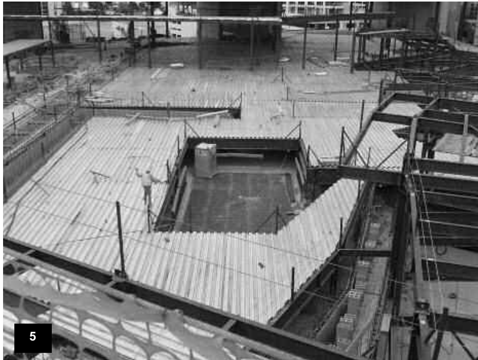
Podium Pool Deck – View of the structural steel framing and metal decking with pool openings framed.
