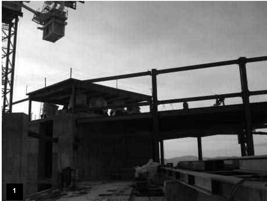
Tower Roof - View of the roof top dunnage steel for the roof top HVAC units, vertical steel for the curtain wall system parapet and the elevator penthouse.
