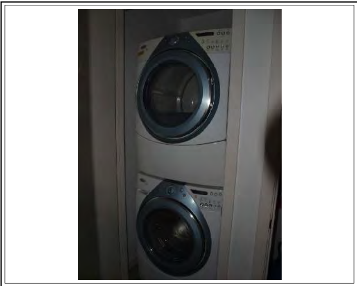
First floor washer/dryer cabinet.
