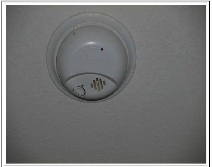
One of many combination CO and smoke alarms.
